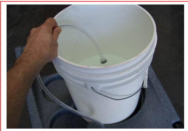
Place Chemical Feed Hose into Rinse Solution
